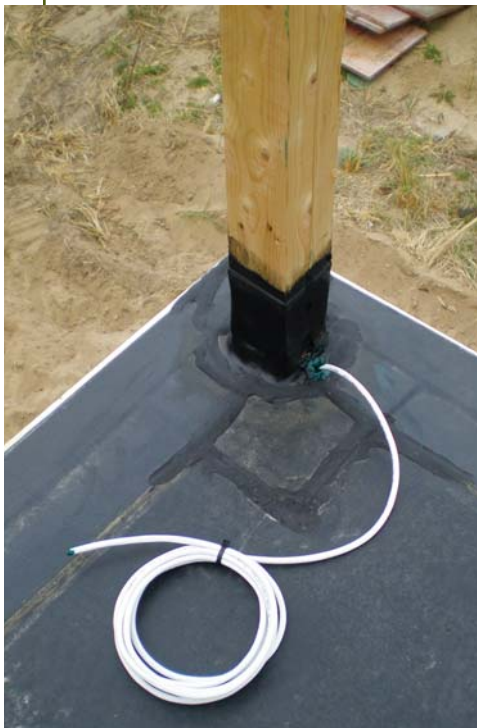
Figure 4. When the deck is above a waterproofed room below, it's important to schedule the audio installer in before the roofer to ensure the wire penetrations are waterproof.
