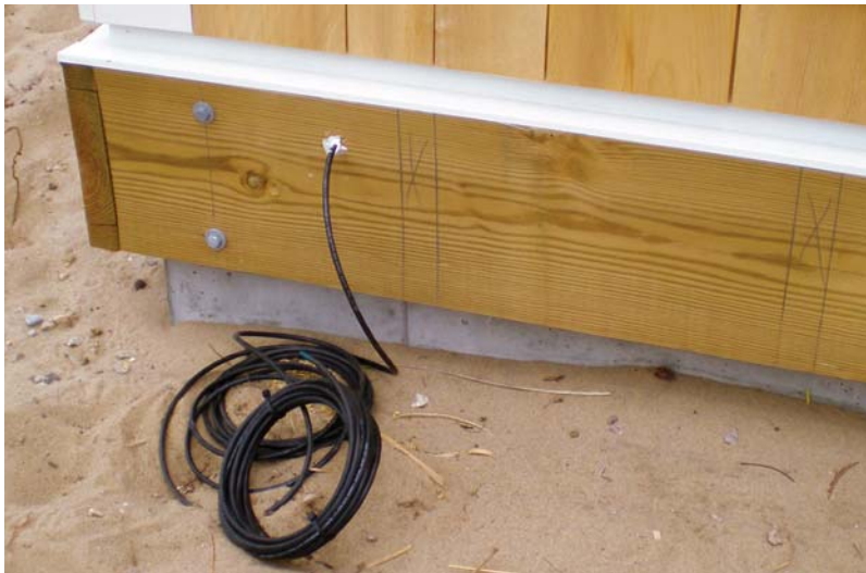
Figure 3. The author usually pulls the speaker wire through a hole drilled in the ledger before the deck is framed and leaves a long length coiled and ready to be run to the speaker locations.
